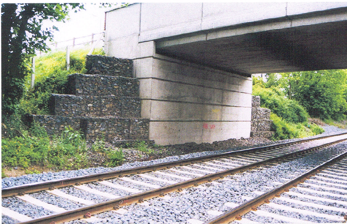
Figure 7.6 Modern re-inforced concrete bridge at Lambeg, NIR. Detail of one abutment. Note the use of rock filled gabions rather than wing walls.
